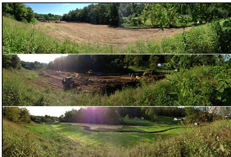
Before, during and after views of the Grave Creek mitigation site east of Cameron, WV developed as mitigation for a construction project. Resource Environmental Solutions, LLC Photo.
