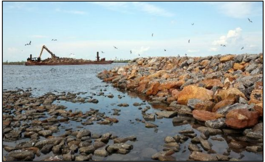
Construction of a rock dam closure for the MRGO channel. Photo taken in 2009 by Bob Marshall, The New Orleans Times-Picayune .
